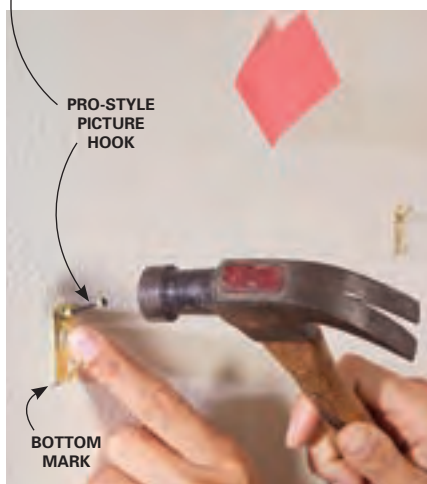
5 Align the bottom edge of a picture hook with the mark and drive a nail through the hook's guide.
